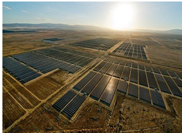
Raghanseda Solar Park, Banaskantha District, Gujarat
