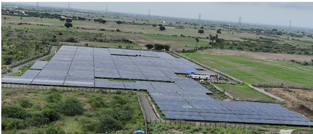
Ground-mounted solar installation for Dalmia Bharat Green Vision Limited in Sattur, Tamil Nadu
