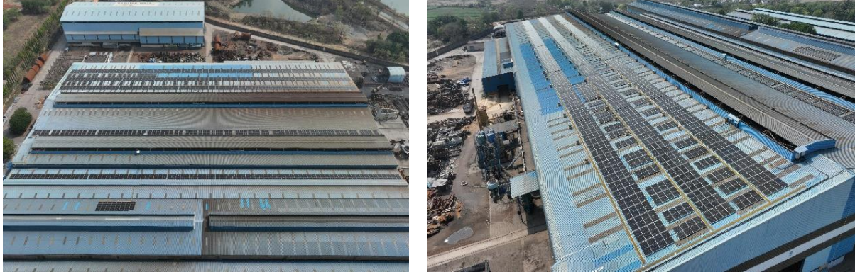
Rooftop solar installation for Jindal Steel and Power Limited in Raipur, Chhatisgarh
