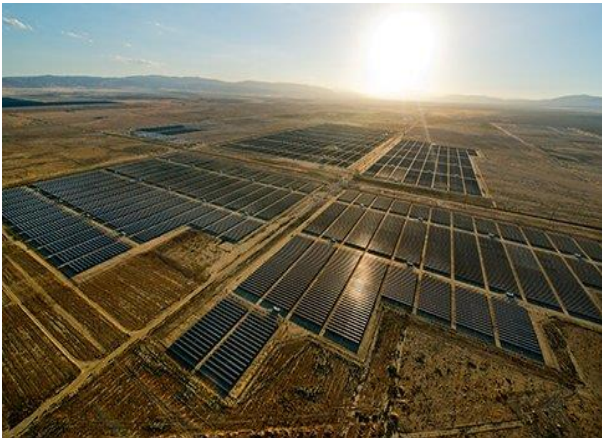
Raghanseda Solar Park, Banaskantha District, Gujarat
